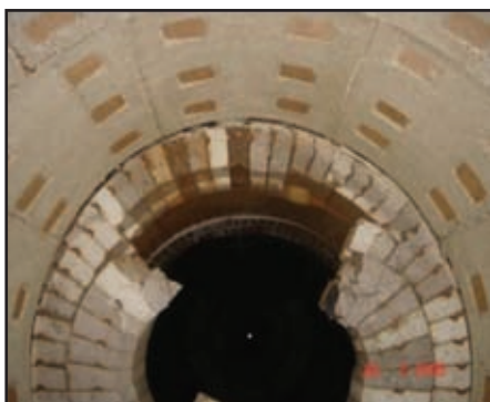
Fig. 2: Furnace choke ring failure due to refractory subsidence
