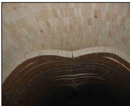
Fig. 1: Hot face layer subsidence
